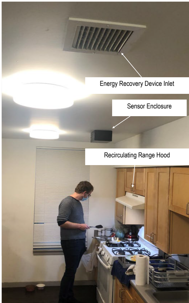
IAQ sensor installed in kitchen with an energy-recovery ventilator.
