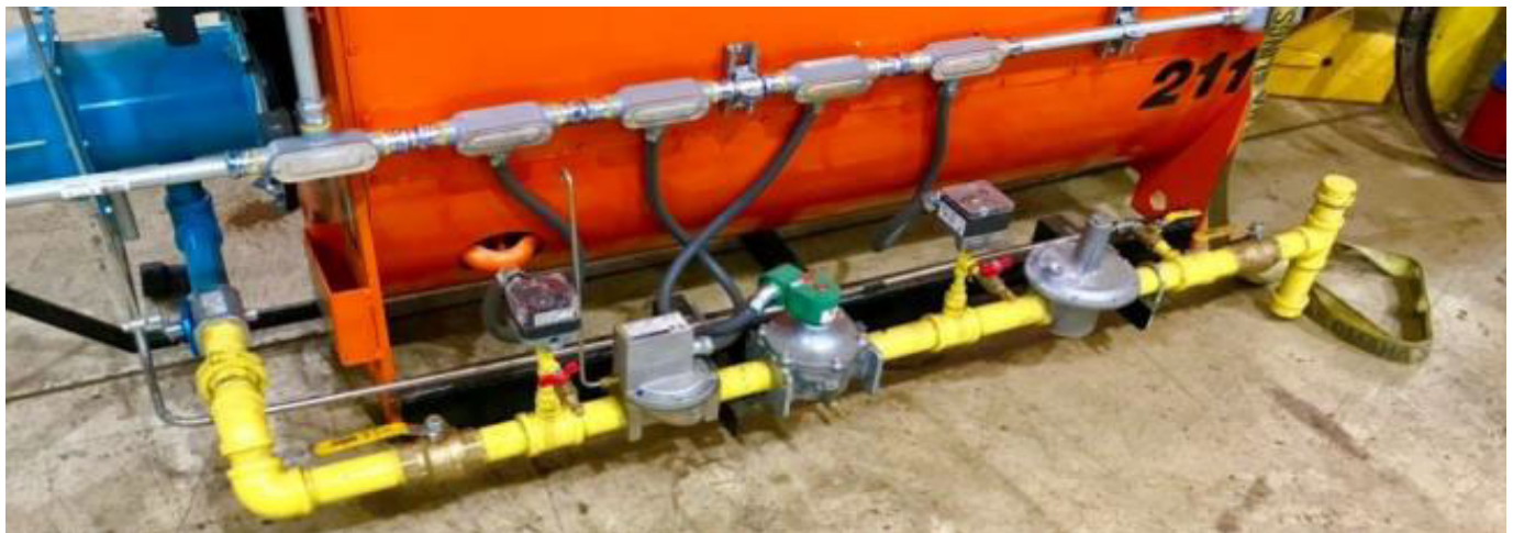
Example Boiler Gas Train (credit: Dungs)
