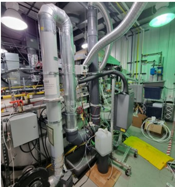
The regenerator tower
