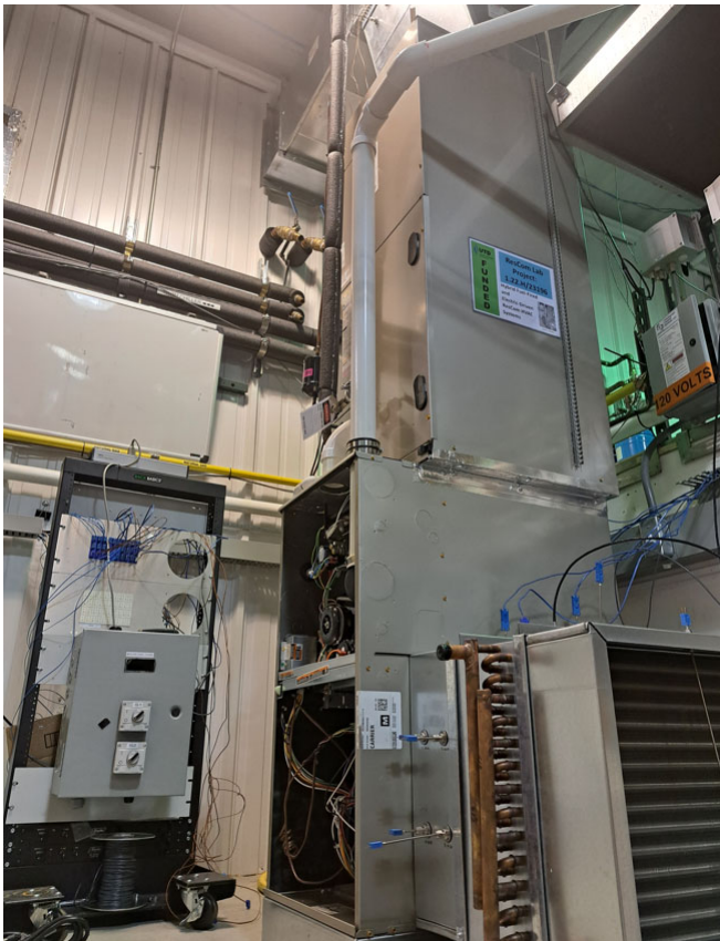
Simultaneous hybrid/dual fuel heating system in laboratory test stand
