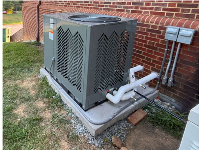
Heat pump outdoor unit installed.
