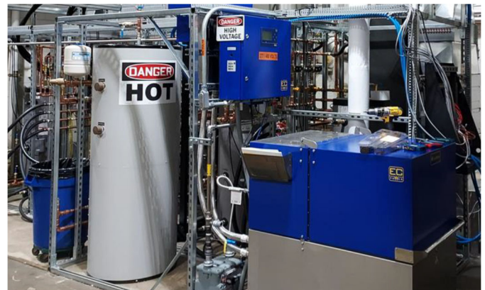
The mCHP integrated system indoor installation.
