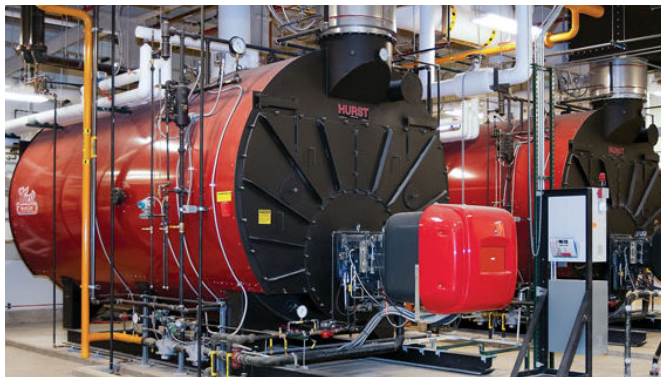
Example of an industrial boiler installation. Image Credit: Hurst Boiler and Welding Inc.
