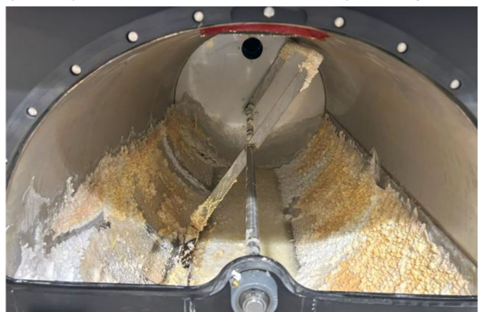
Interior of reaction chamber after operating unit for a few hours with ~25 kg of caustic potash
