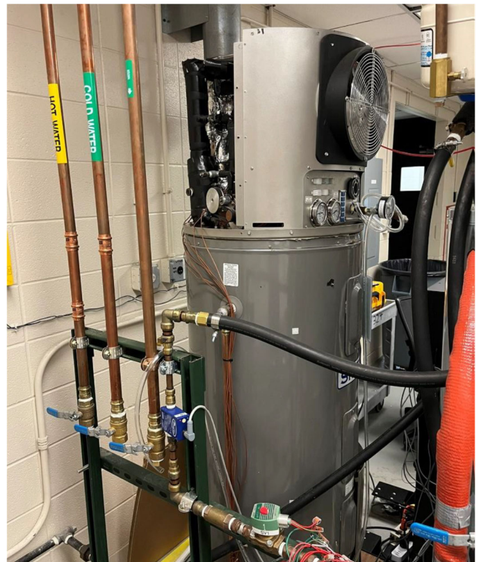
GHPWH Prototype Unit Installed in Laboratory
