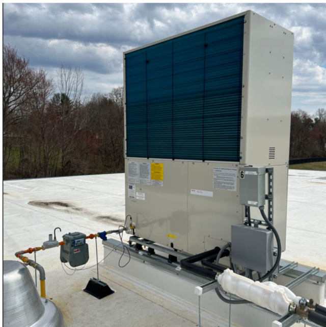
Example of a Yanmar Gas Engine Heat Pump being analyzed, with a gas meter to monitor gas consumption
