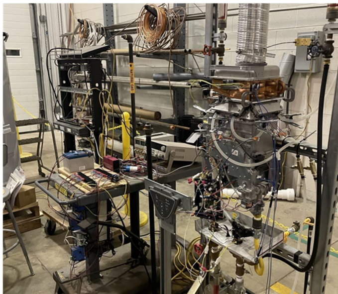
TEG integration and testing with the tankless water heater
