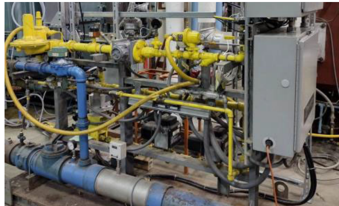
Air-fuel skid assembly for H2 operation
