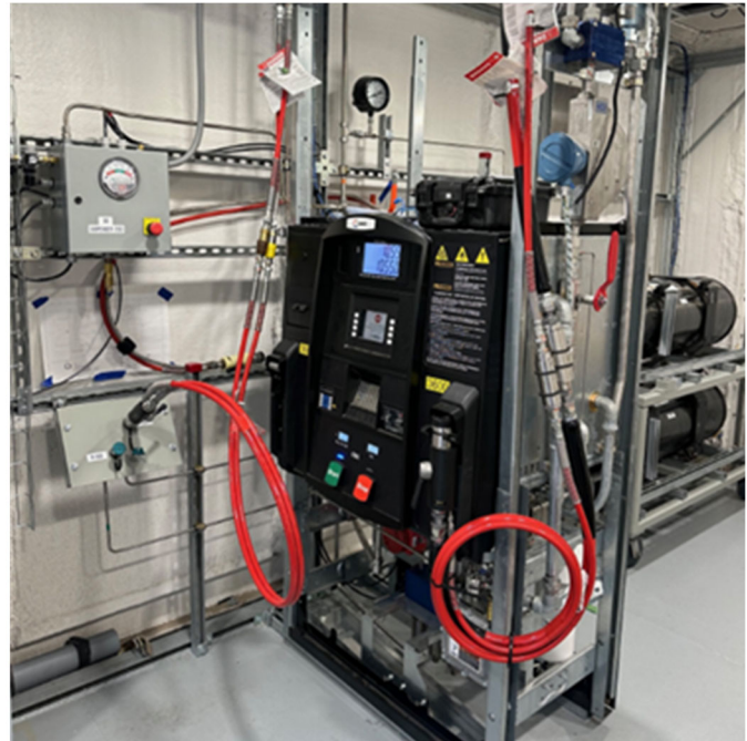
The fully installed ANGI dispenser
