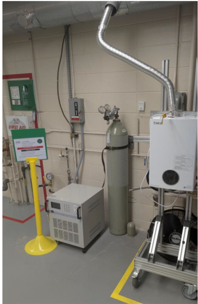
Laboratory Stand to test Singapore appliance being commissioned
