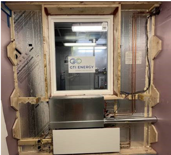
Hydronic Shell envelope/mechanical panel
