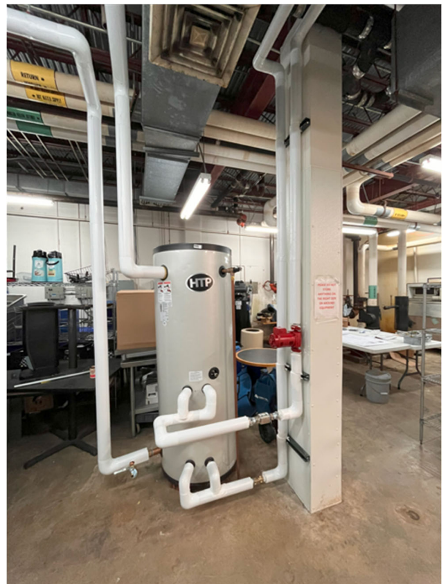
Indoor indirect water heating tank plumbed in parallel with the existing water heating loop.
