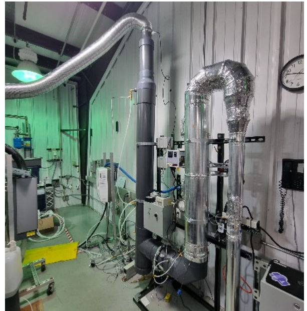
The conditioner tower
