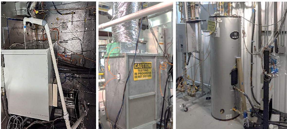
Prototype GAHP hybrid (left) and paired prototype air-handling unit (right).
