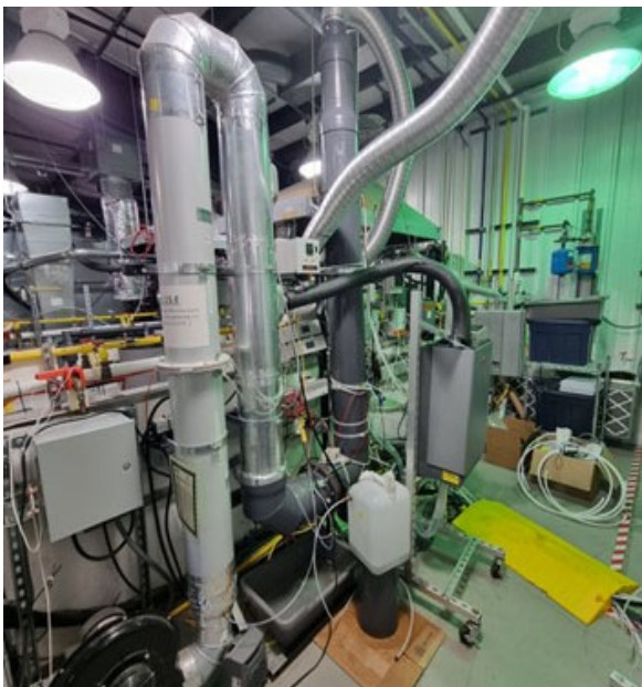
The regenerator tower
