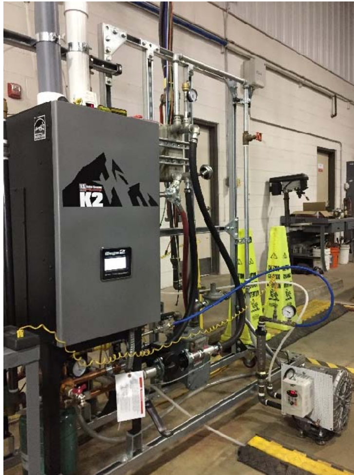
Figure 10. Flue Gas Recycle Test Set-Up
