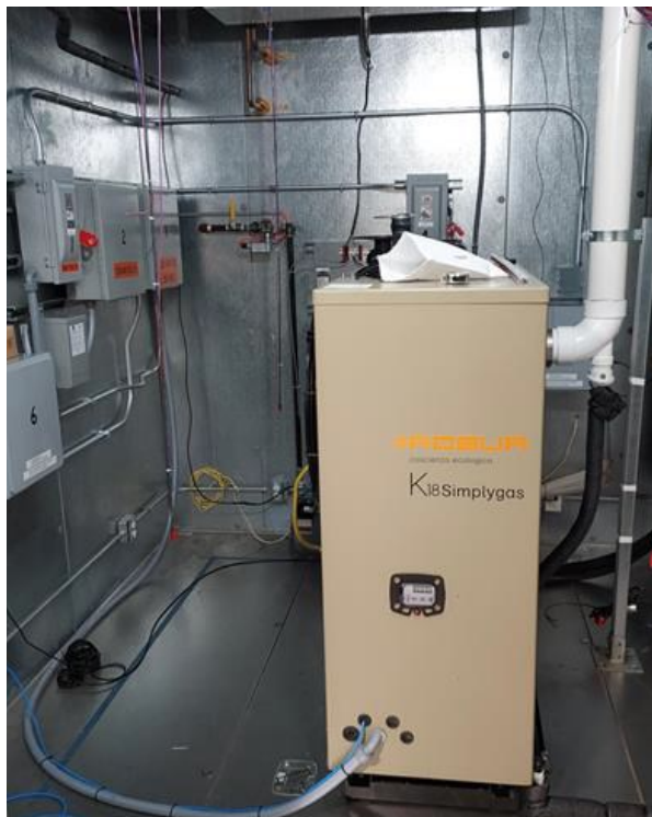
A prototype North American Robur K18 GAHP installed inside a laboratory environmental test chamber
