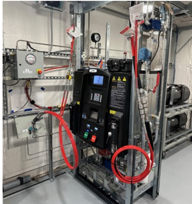
The fully installed ANGI dispenser
