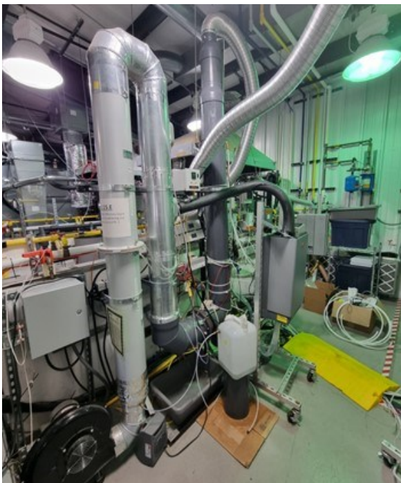
The regenerator tower
