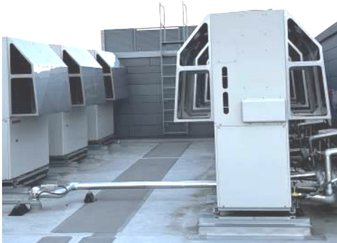
Seven installed GHPs at the host site in Dover, DE.
