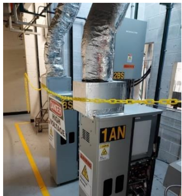
AISIN SOFCs installation at research laboratory
