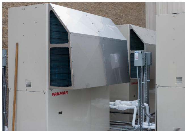
One of six GHPs installed at the Lawrenceville Public Works facility in Georgia.
