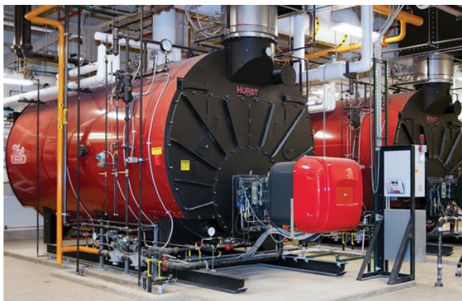
Example of an industrial boiler installation. Image Credit: Hurst Boiler and Welding Inc.
