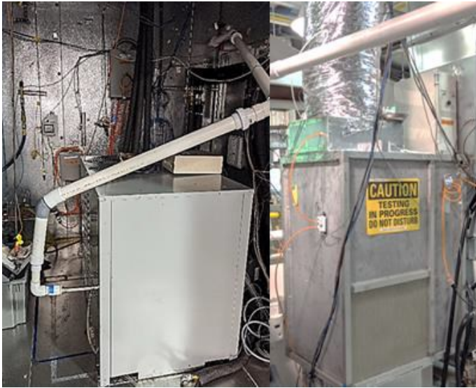
SMTI 40K Hybrid GAHP system installation in HVAC laboratory. (left) The installation of the GAHP in a environmental chamber; (right)
