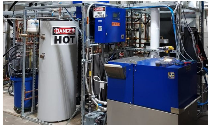
The mCHP integrated system indoor installation.
