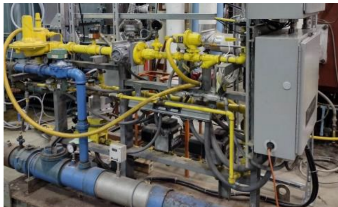
Air-fuel skid assembly for H2 operation
