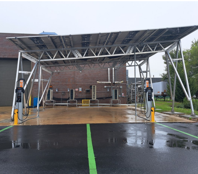
The mCHP integrated system outdoor installation.
