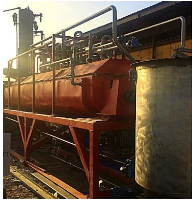
Thermo-Vacuum Dryer of 100 tons per day capacity in previous UTD project 2.17.B
