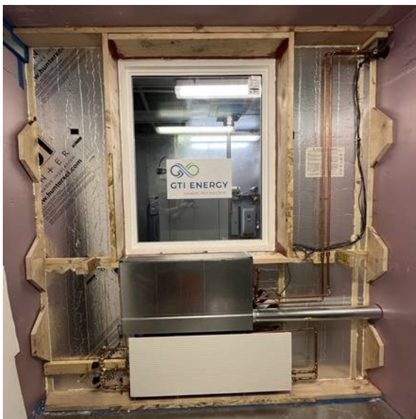
Hydronic Shell envelope/mechanical panel
