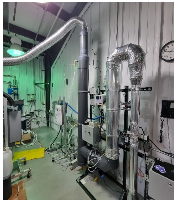
The conditioner tower
